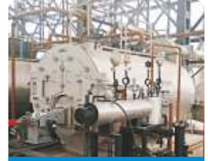
OIL FIRED PRESSURIZED HOT WATER GENERATOR
