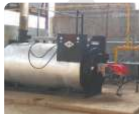
FUEL OIL FIRED THERMAL OIL HEATING SYSTEM
