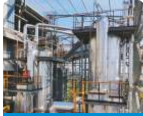
COAL FIRED HIGH PRESSURE THERMOSYPHON
