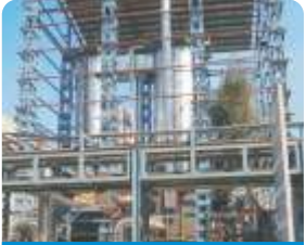
COAL FIRED FBC THERMAL OIL HEATING SYSTEM
