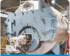
HEAVY OIL FIRED STEAM BOILER
