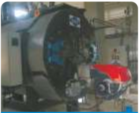
GAS FIRED STEAM BOILER
