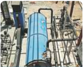
FUEL OIL FIRED THERMAL OIL HEATER
