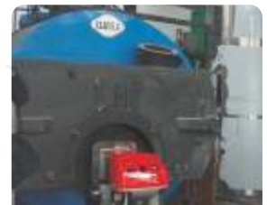
DIESEL FIRED STEAM BOILER
