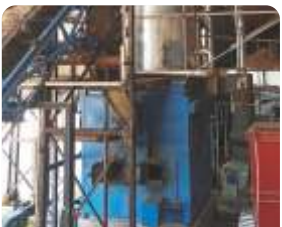
BAGASSE FIRED HIGH PRESSURE THERMOSYPHON
