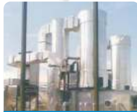
BIOMASS FIRED THERMAL OIL HEATER SYSTEM
