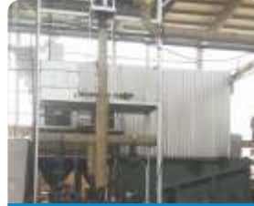
BIOMASS THERMAL OIL HEATING SYSTEM
