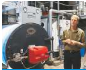
FUEL OIL FIRED THERMAL OIL HEATING SYSTEM
